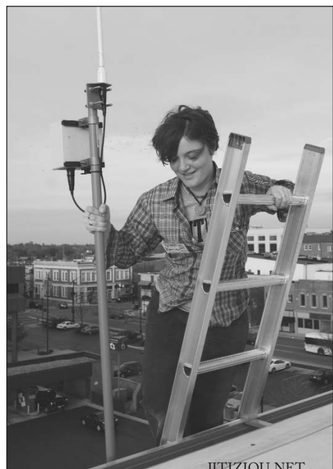
Volunteer, Katie Kenlan, carries the wifi node and antenna to the top of the Library in downtown Urbana.
